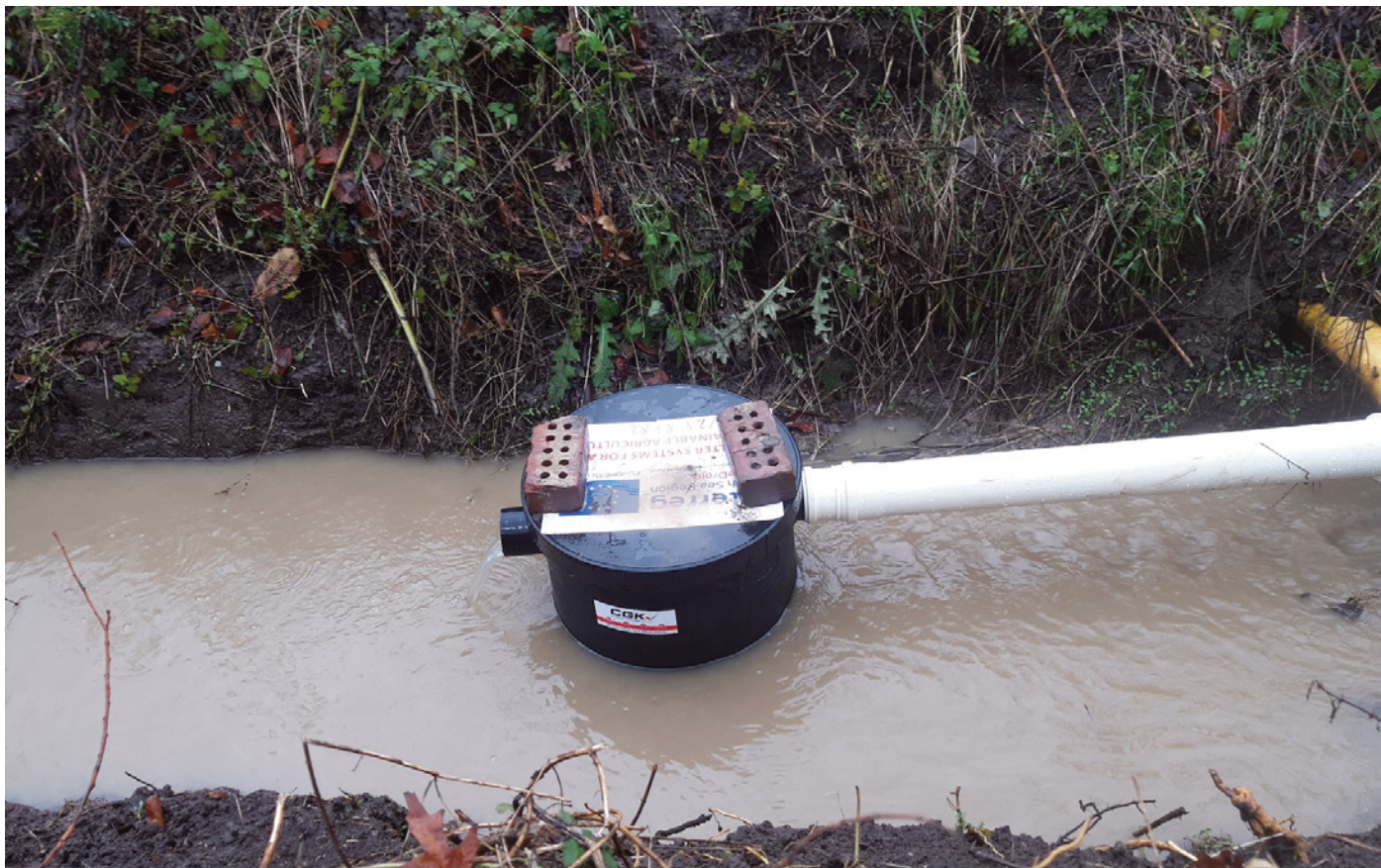
Fig. 1 A phosphorus filter box is directly connected to a tile drainage pipe. The filter box is filled with iron-coated sand (ICS), which adsorbs phosphate and lowers the phosphorus concentration in the ditch water
